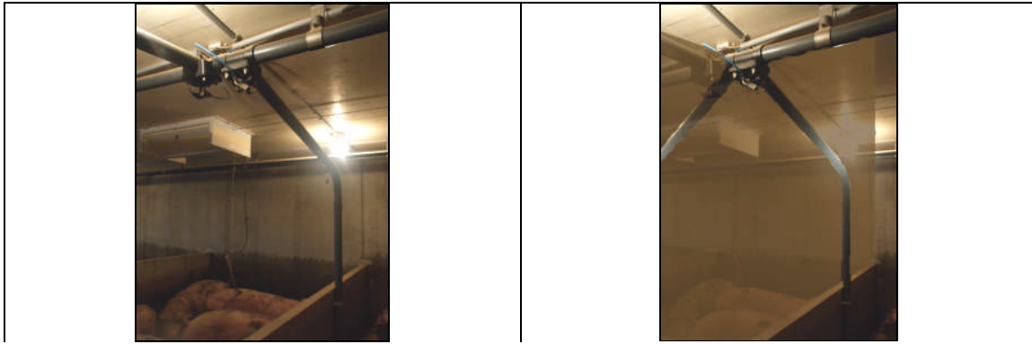
The 120 finishing room can be easily divided into two airspaces needing a wall and a Y piece on the feederline
